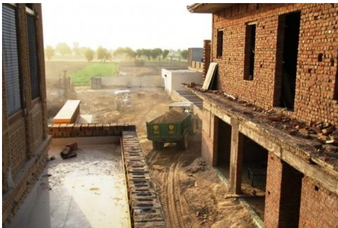
After laying the foundation of the staff residences, tractors haul in dirt to fill in area. The dirt-movers came at dusk and worked some hours in the dark
